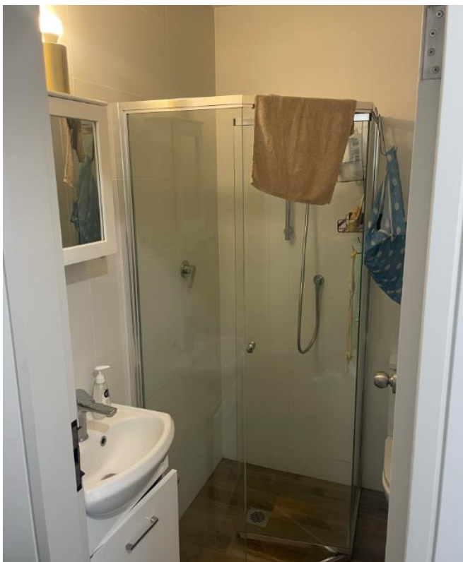
Figure 11: Former kitchen which has been converted into three separate bathrooms without development consent
