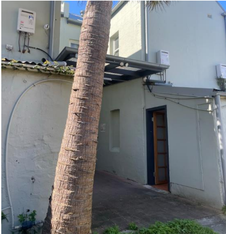
Figure 4: Photograph showing skillion addition to rear (right-hand side of photo) which is proposed for demolition and existing cabbage tree palm located within the adjoining site at 193 Harris Street
