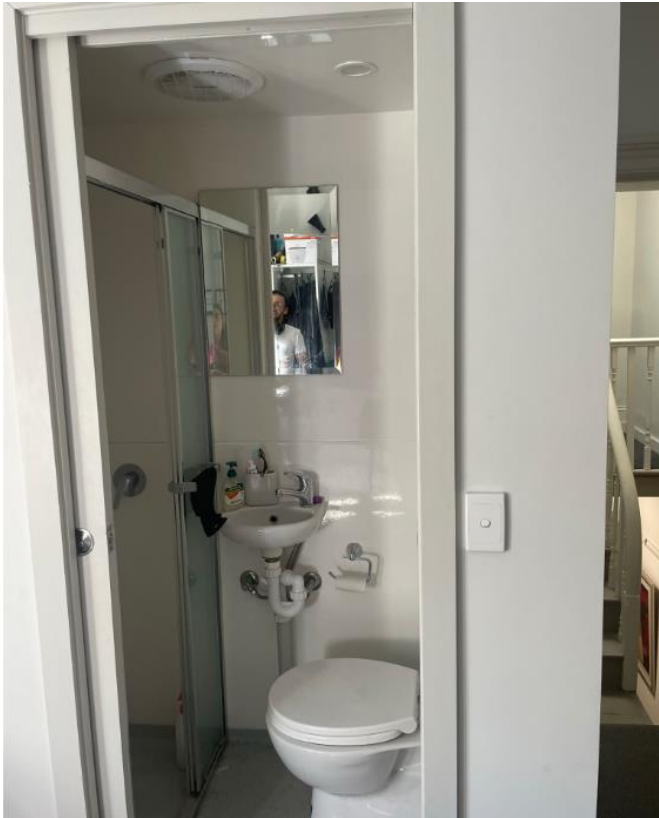
Figure 12: Room 5 with ensuite bathroom constructed without development consent
