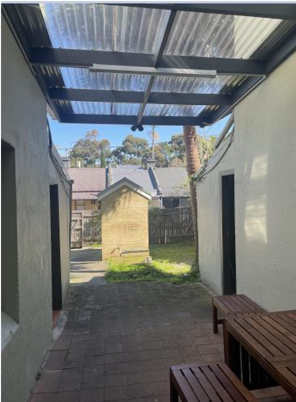
Figure 3: Ground floor rear wings of Nos. 195 (left) and 193 (right), noting 193 and 195 Harris Street share a communal open space at the rear
