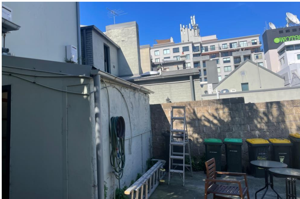
Figure 5: Photograph showing skillion addition (proposed for demolition) abutting adjoining development at 197 Harris Street
