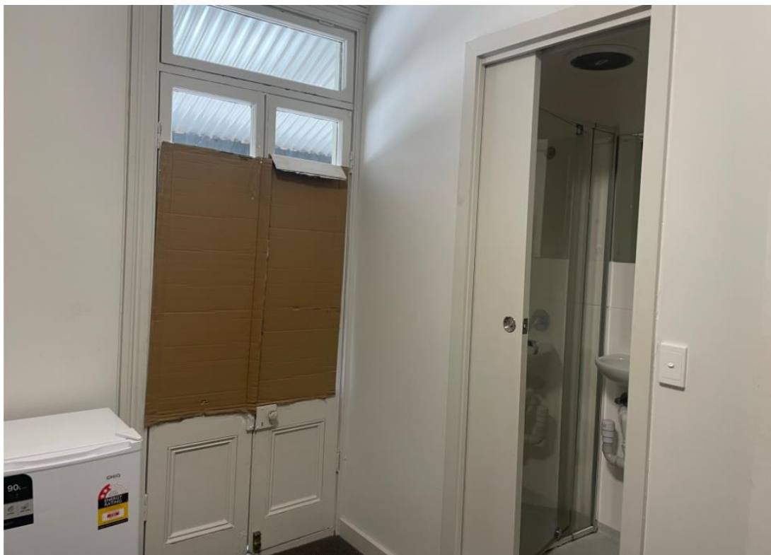
Figure 13: Room 3 with ensuite bathroom constructed without development consent
